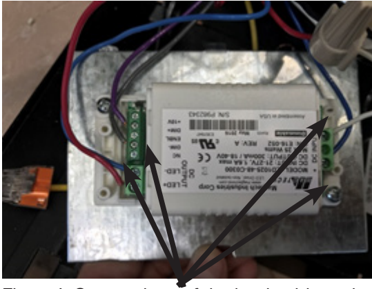
Figure I: Connections of the load cable and the ESCD1000 to the LED Driver.
