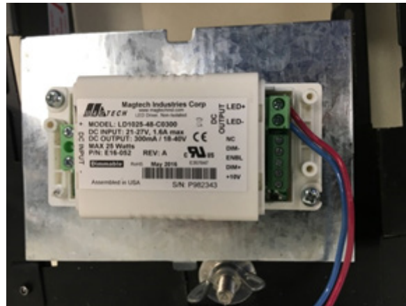
Figure D: Covers are removed from the LED driver to expose the Dimming and Power connections
